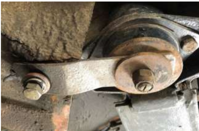
Loose bolt on the left
