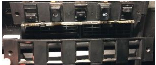
Figure 2 – panel cover removed
