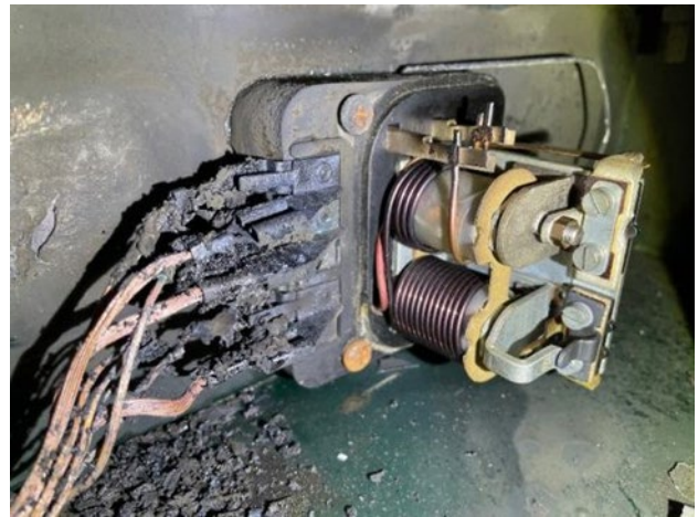
Voltage regulator is a bit more worse for wear
