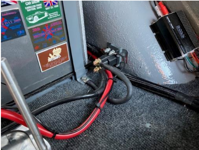
Relay connected for the test
