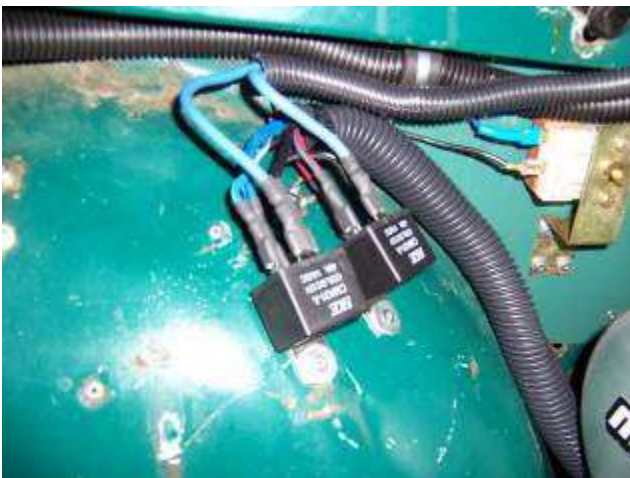
Figure 4: 40 Amp Relays On The Inner Fender, No Direct Switching Here
