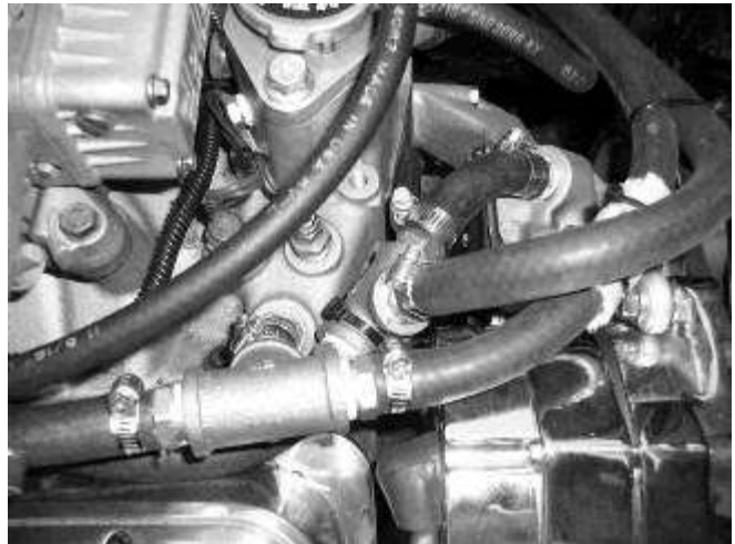
Mess Of Extra Plumbing I Had To Install For The Aux Cooler – Thank Goodness Lowes Is Open Until 10PM!
