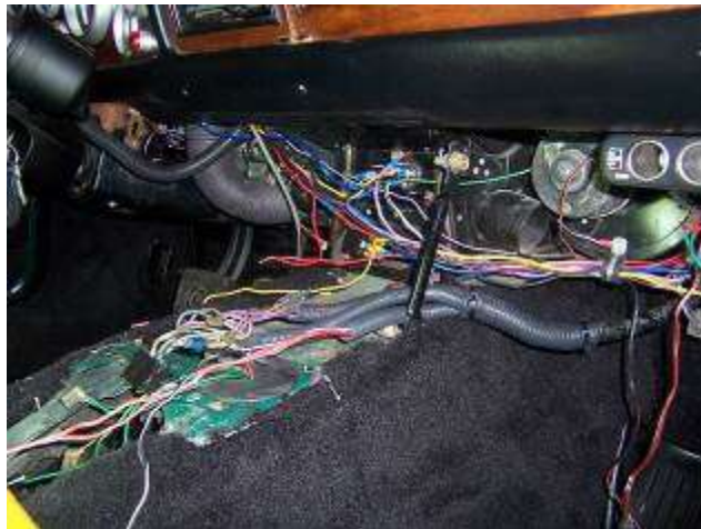
Wiring Mods About Half Way Through – Messy, Messy, Messy.
